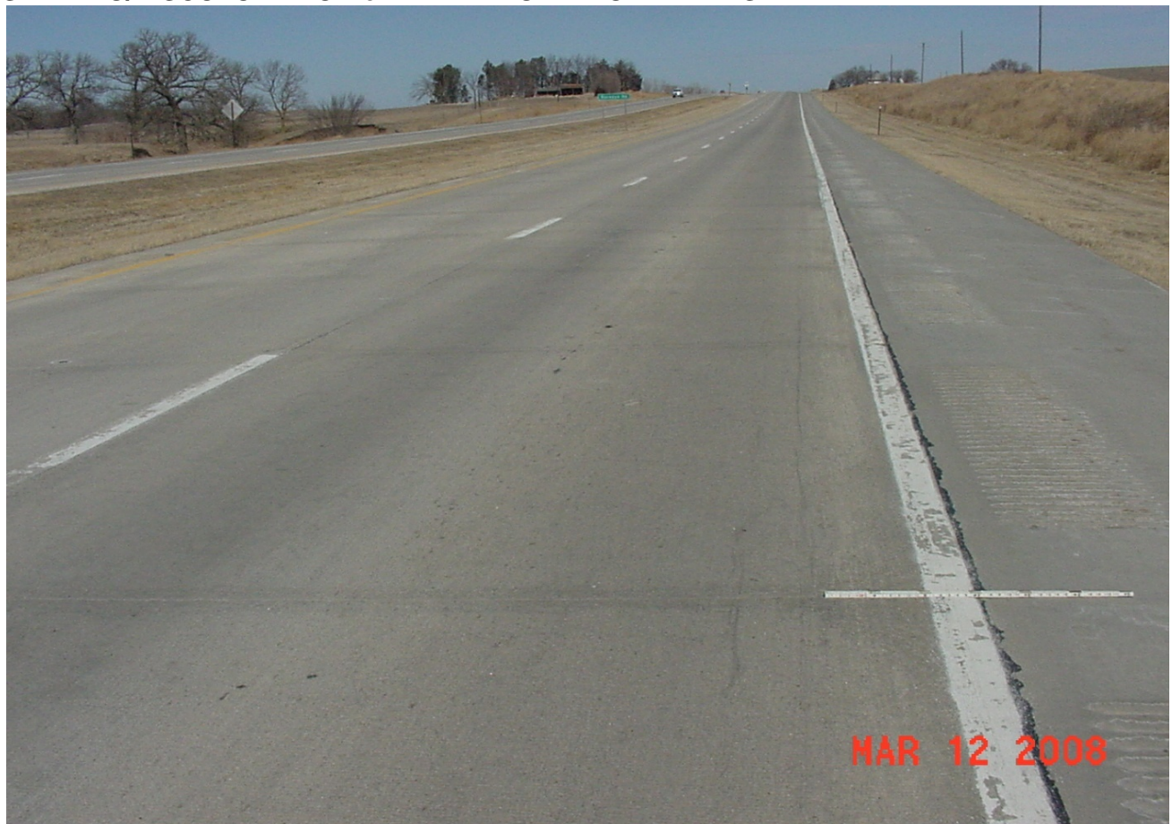
STAINING/DISCOLORATION on LANE EDGE – MODERATE SEVERITY
