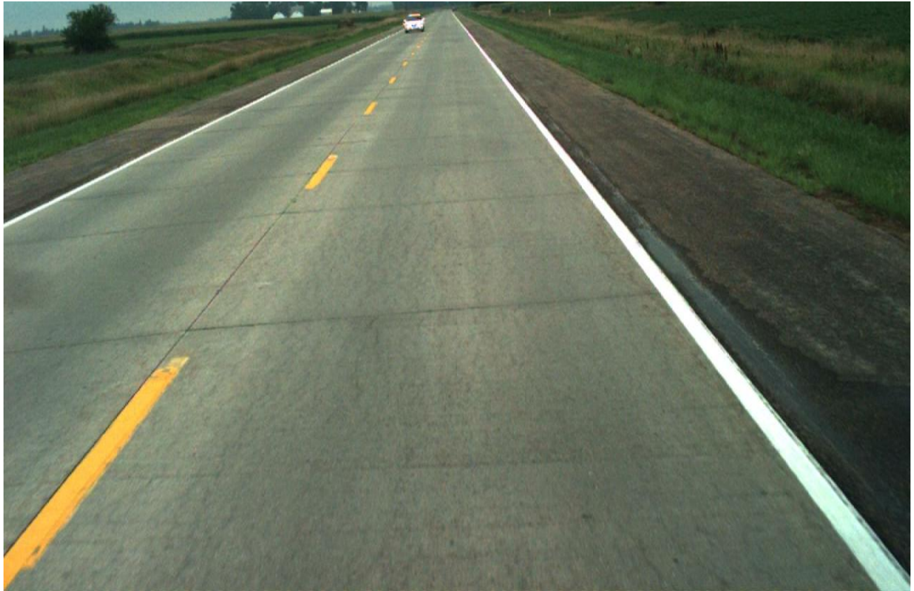
RANDOM STAINING/DISCOLORATION with CRACKING – MODERATE SEVERITY
