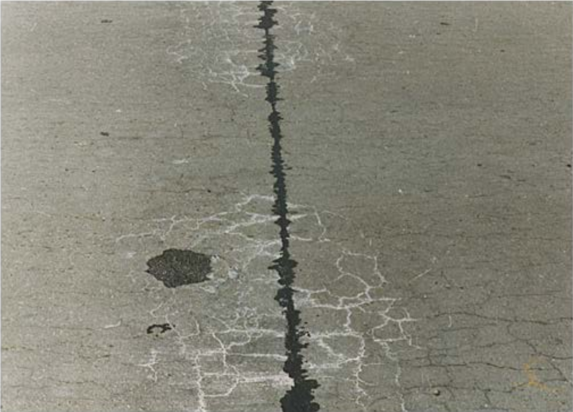
REGULAR JOINT - HIGH SEVERITY
