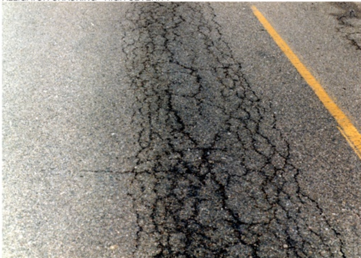
ALLIGATOR CRACKING - HIGH SEVERITY
