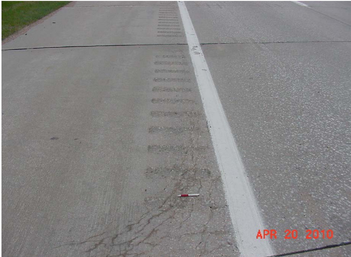
SHOULDER CONDITION – LOW DISTRESS
