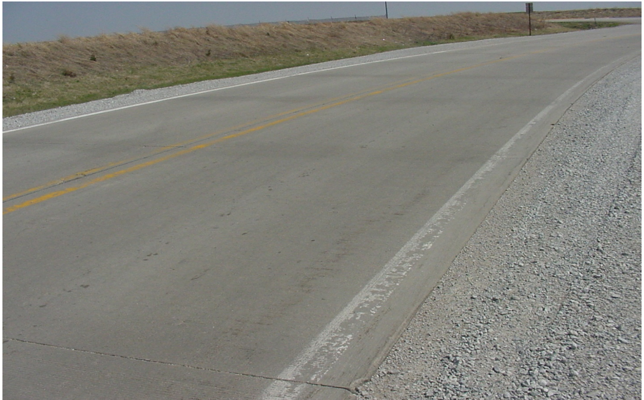
REGULAR JOINT – STAINED MODERATE SEVERITY
