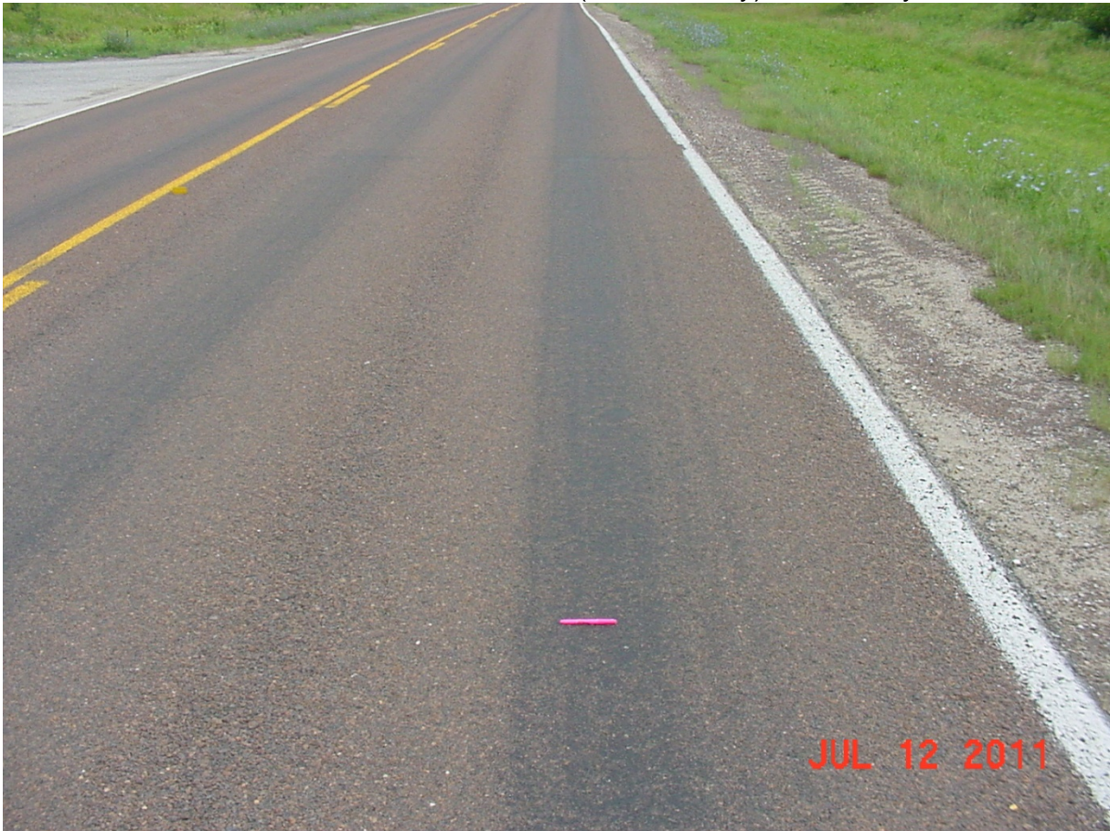
EXCESS ASPHALT on Armor Coated Road (Low Severity) Added July, 2011
