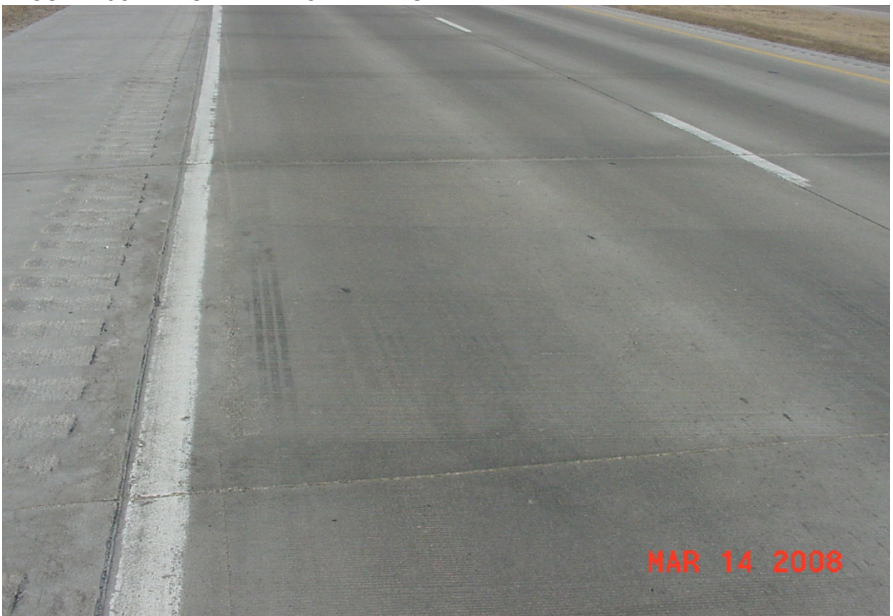
REGULAR JOINT – STAINED MODERATE SEVERITY
