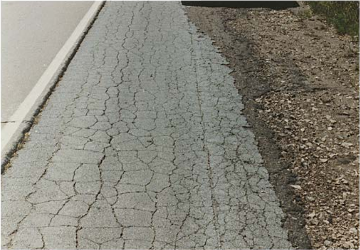
SHOULDER CONDITION – HIGH SEVERITY
