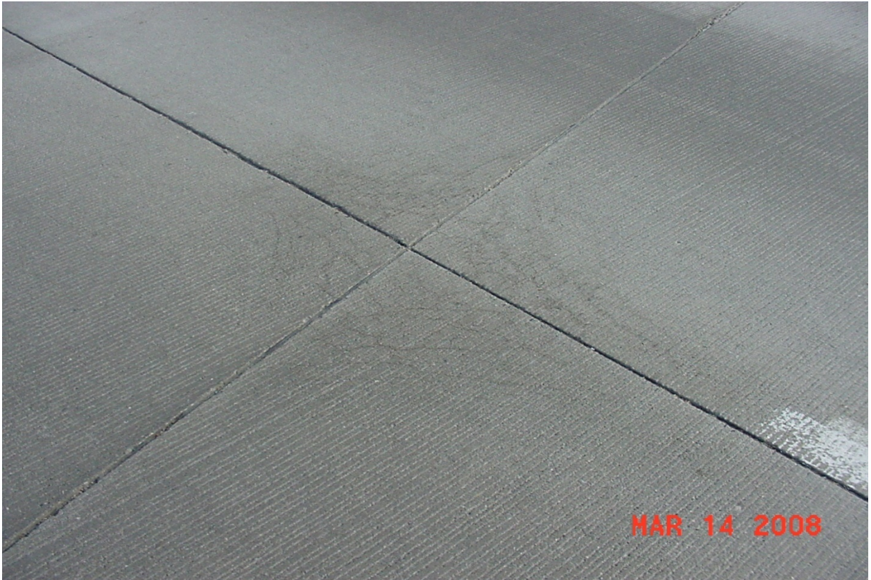
REGULAR JOINT – STAINED AND CRACKED MODERATE SEVERITY
